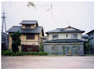
Photo 2. Adjacent houses tilted towards inside.
